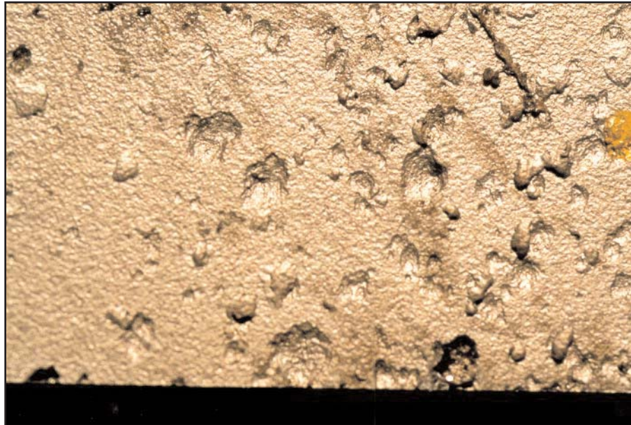
Figure IX-15: Iron Oxide Corrosion Products Removed to Reveal Depressions
