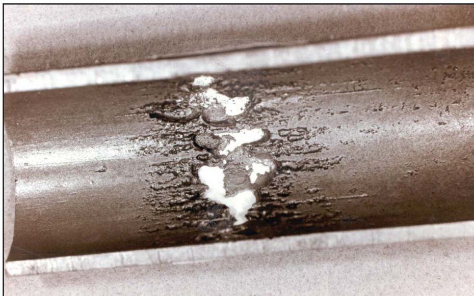
Figure I-18: Suspected Ringworm Corrosion
