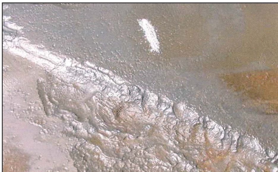
Figure VIII-13: Close-up View of the Corrosion at a Plate Boundary
