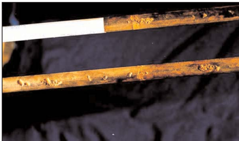
Figure IX-38: Scattered, Deep External Surface Depressions
