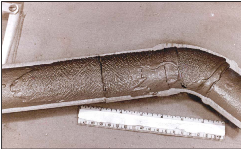
Figure I-42: Severe Metal Loss in Bend
