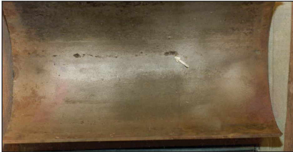
Figure IV-9: MIC Detected in the 3 o'clock Position
