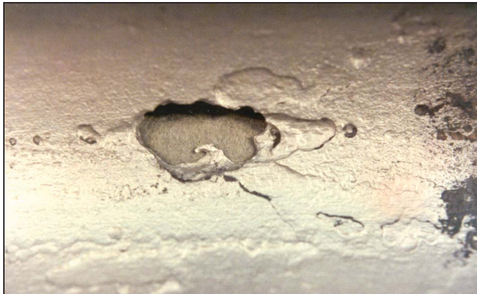
Figure I-11: Tubing Perforated by CO 2 Corrosion
