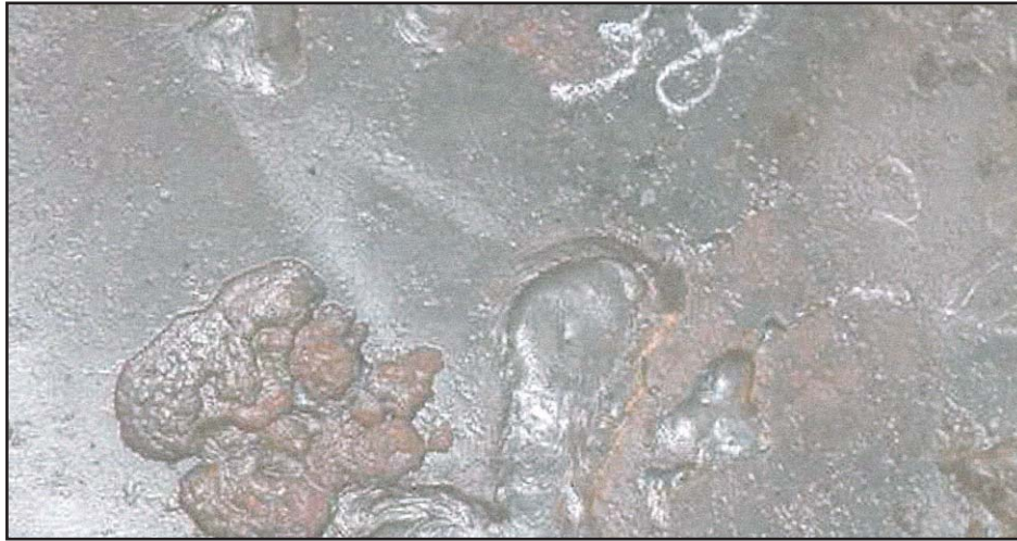
Figure VIII-14: UAN Corrosion on Carbon Steel Storage Tanks
