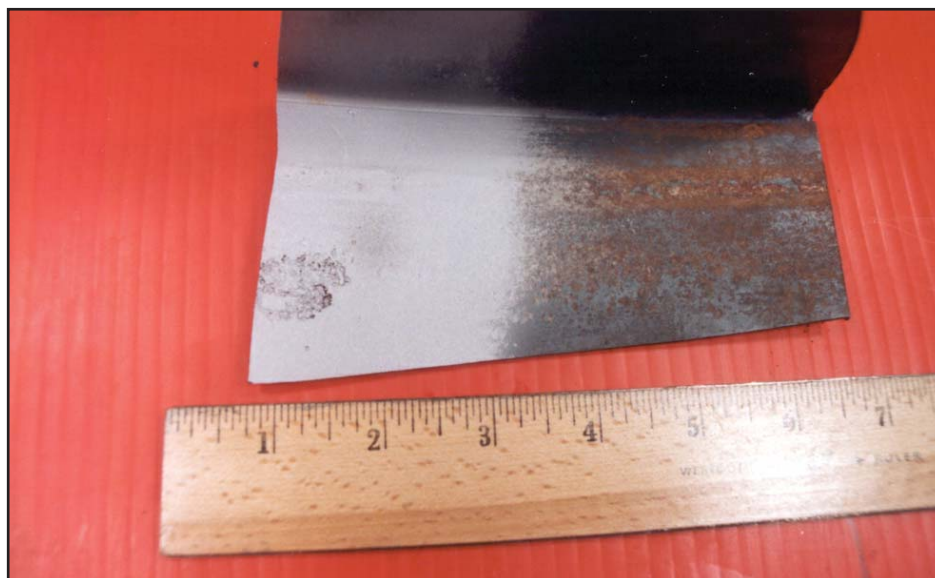
Figure VIII-15: Fuel Storage Tank Corrosion
