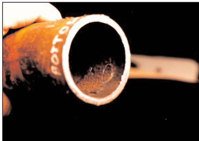
Figure IX-18: Localized Deposition at Bulge Site
