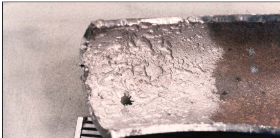
Figure I-43: Flow-Enhanced Corrosion in U-bend
