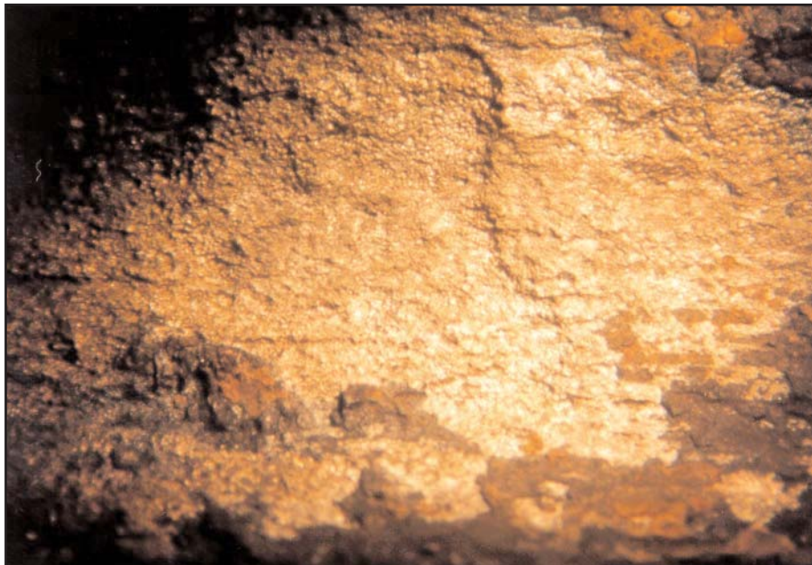
Figure IX-42: Deposit and Corrosion Product Layers Removed to Reveal Rough-surfaced, Undercut Depressions
