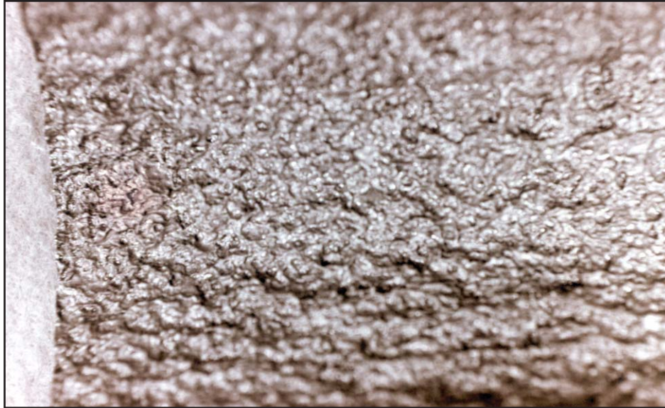
Figure I-5: Uniform Corrosion Showing Hills and Valleys
