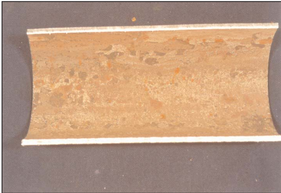
Figure IX-9: Heavy Deposit Layers Covering Internal Surface of Boiler Tube
