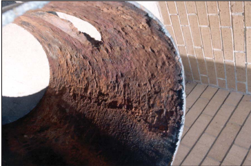
Figure V-1: Hydrochloric Acid and Hydrogen Sulfide Corrosion
