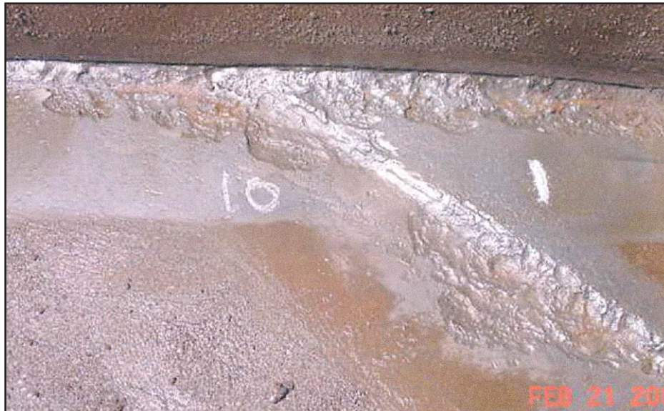
Figure VIII-12: UAN Corrosion — Carbon Steel Storage Tank
