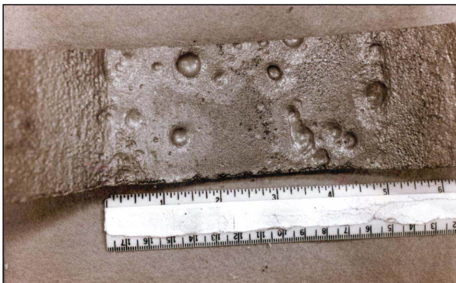
Figure II-2: Oxygen Corrosion in a Flowline
