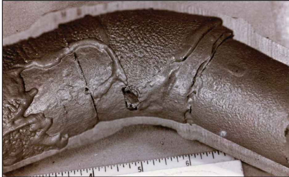
Figure I-41: Combination of Corrosion Mechanisms
