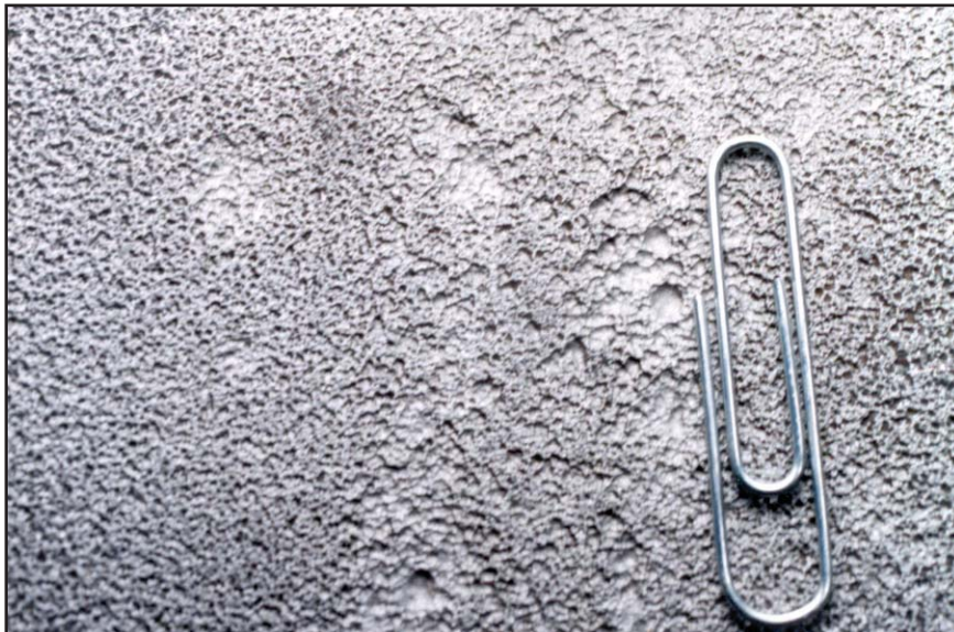
Figure VIII-9: Close-up of Carbon Steel Product Pipeline Corrosion
